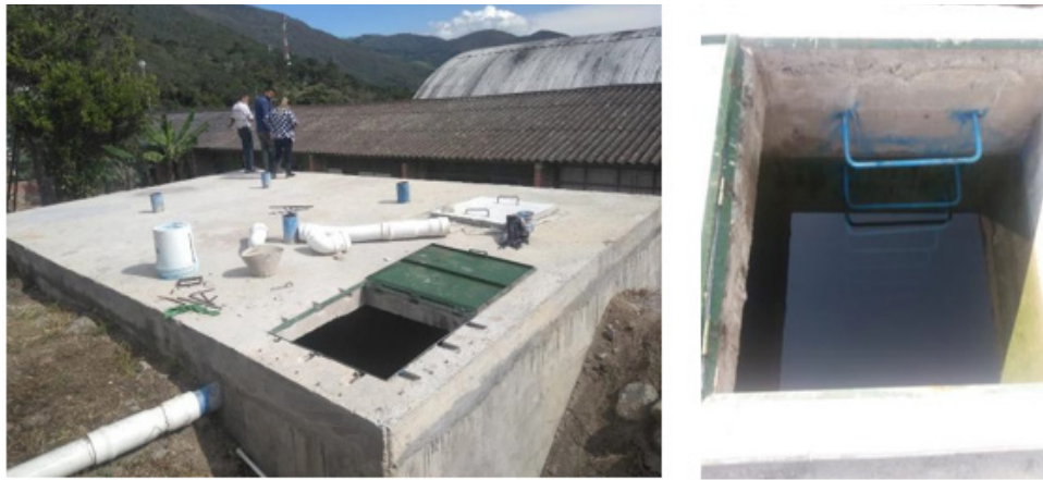
Figure 15. New Storage Tank
