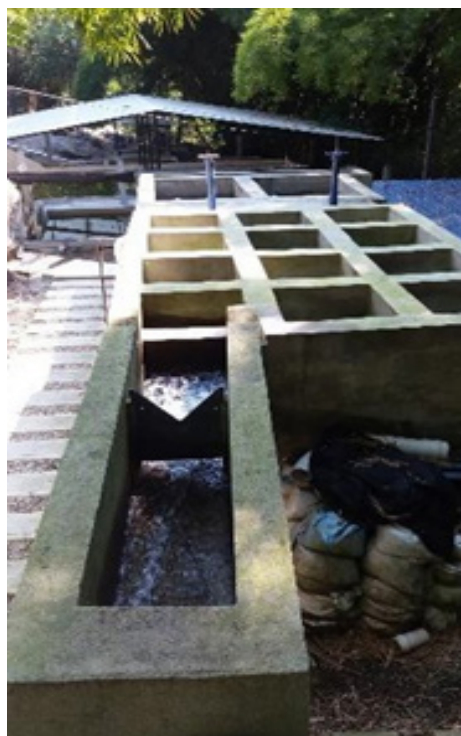
Figure 8. Parshall flume and Alabama type flocculator
