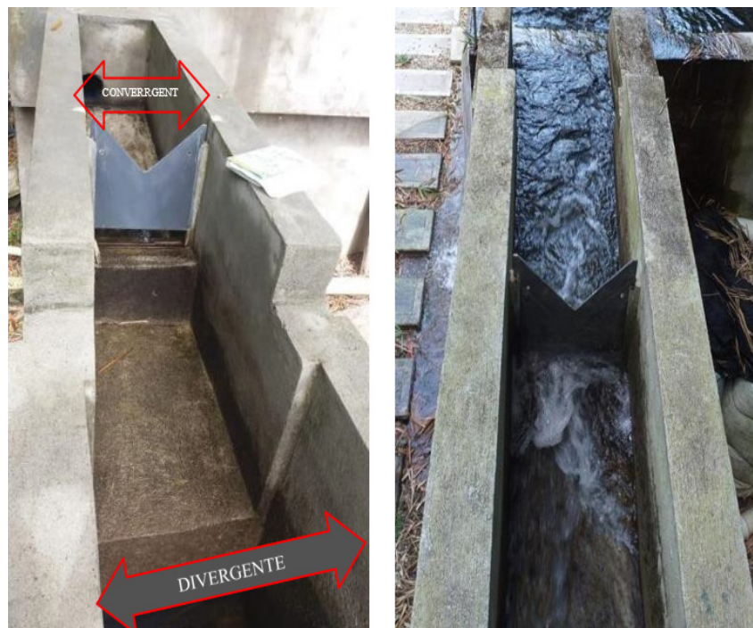
Figure 6. Inlet pipe and Parshall flume
